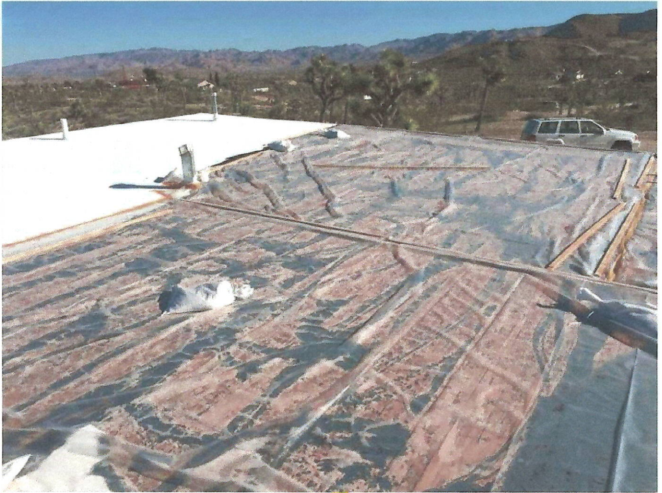
17 16-02-12-2019 015 Date Taken: 2/11/2019 Wind damaged area- temp cover
